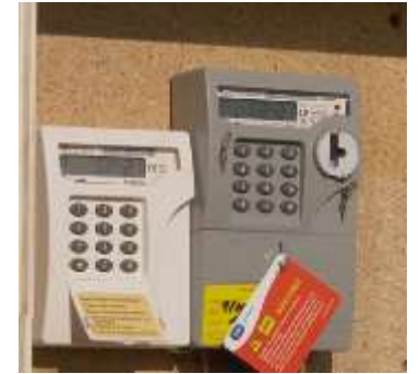
Electricity access universal; but equality issues remain
