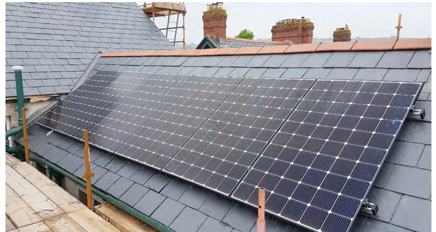
PV array in Aldworth
